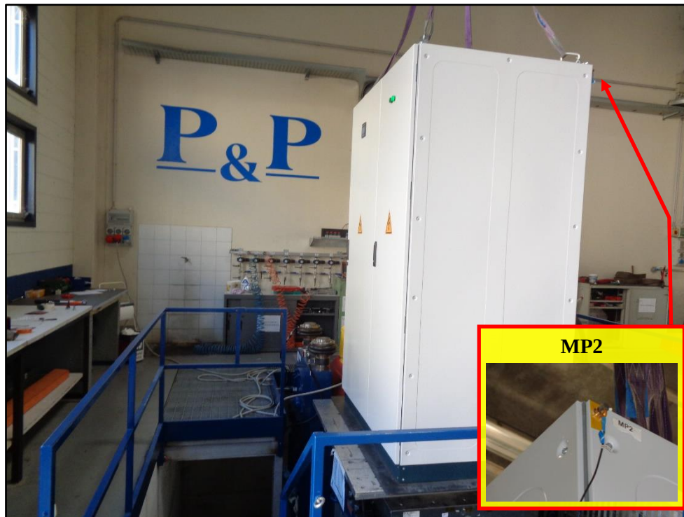
Photo 7 - Measuring points on the unit (MP2)
