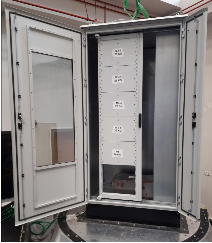
Picture 12. Front View – Doors Open
