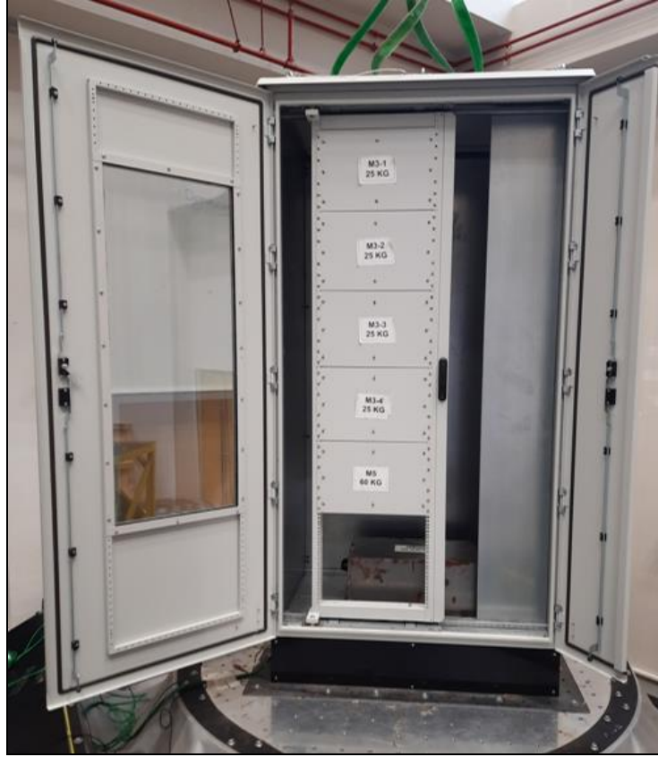
Picture 3. Front View – Doors Open
